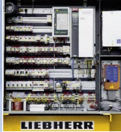
The switchgear cabinet.
